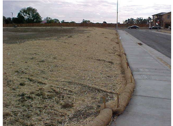
Here is an effective combination of sediment and erosion control using fiber rolls and mulch.
