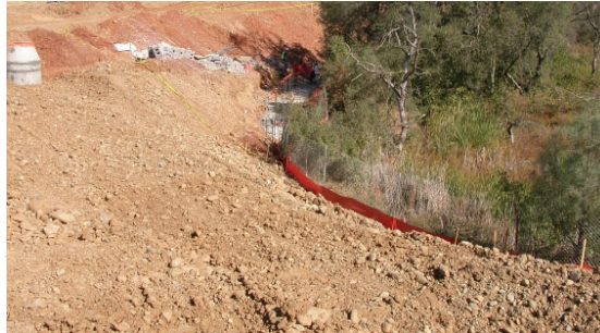
At this site, the silt fence (sediment control) is being used, however; erosion control is also important, especially for steep slopes.
