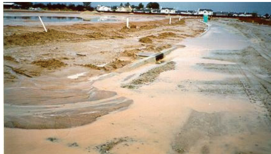
Without proper erosion and sediment control, pollutants such as sediment can enter our local waterways and harm aquatic life.
